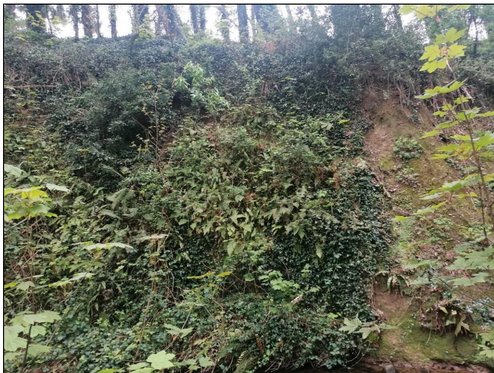
Plate 9. Steep slopes on the southern bank of the river.
