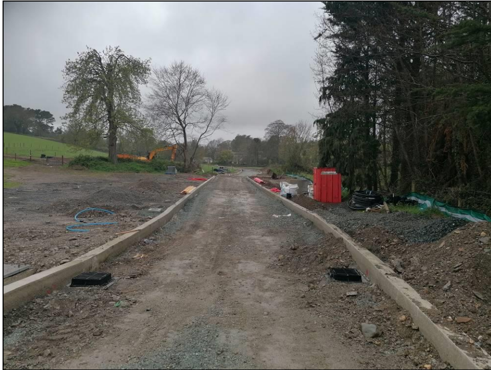
Plate 25. Native woodland planting should be implemented between the construction access road in Oaklawn and the river to create an ecological corridor and protect the river. The land here will need to be rehabilitated prior to planting.
