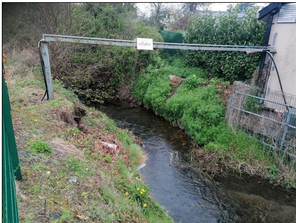
Plate 26. Bare banks at the Castle Inn devoid of vegetation following recent construction works and collapsing as a result.
