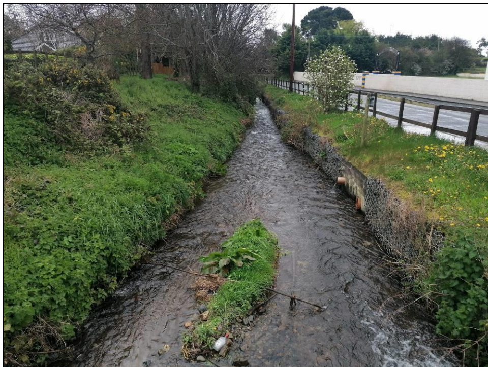
Plate 19. Canalisation of the river beside the Sea Road and installation of rock gabions.
